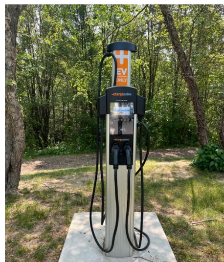
Photo 3: Electric Charging Station.
